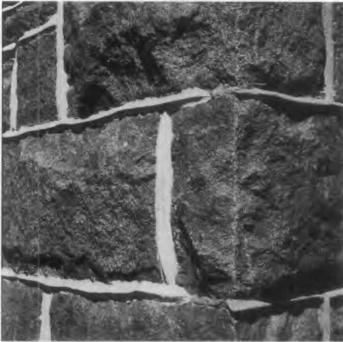
Figure 15. The profile of the repointed joints on the left replicate the historic joints around the corner to the right on the front of this stone building in Leesburg, VA. The contractor's pride in the repointing work is evident by the signature in the vertical joint. Photo: Anne Grimmer.
