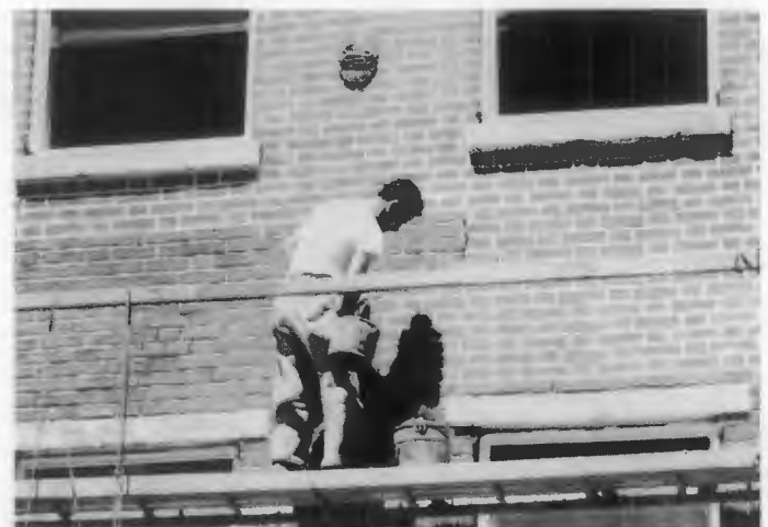
Figure 17. This photograph shows the significant visual change to the character of this historic brick building that has resulted from improper repointing procedures and a noticeably increased thickness of the mortar joints. Photo: Lee H. Nelson, FAIA.
