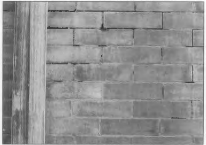
Figure 2. Much of the mortar on this building has been leached away by water from a leaking downspout. The downspout must be replaced and any other drainage problems repaired before repointing. Photo: Robert C. Mack, FAIA.
