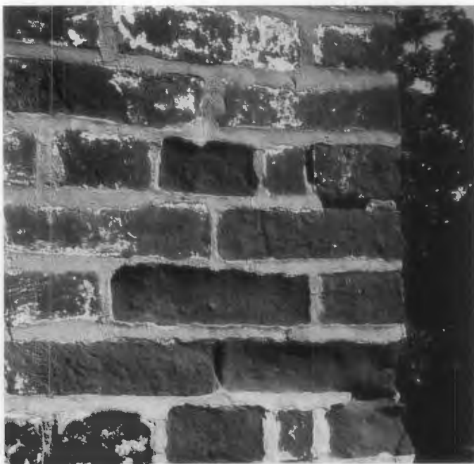
Figure 5. The use of hard, portland-cement mortar that is less permeable than the soft bricks has resulted in severe damage to this brick wall. Moisture trapped in the wall was unable to evaporate through the mortar which is intended to be sacrificial, and thus protect the bricks. As a result the moisture remained in the walls until water pressure eventually popped the surface off the bricks. Photo: National Park Service Files.
